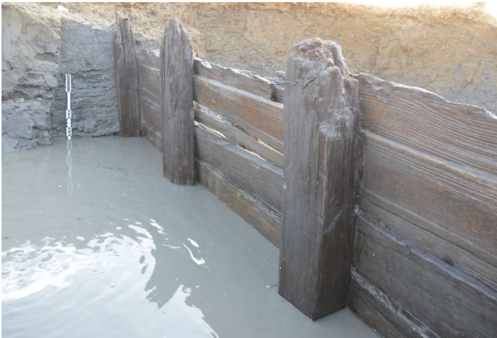
Wooden sheet piling used to build the Mandirac dikes © C. Sanchez, CNRS
